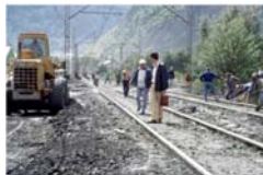
Debris-flows deposition on the international railway France-Italy (1987)
